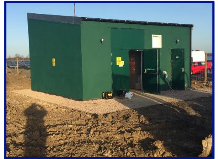
Figure 34: Green DNO Building (Source: Integral Utility Services)
